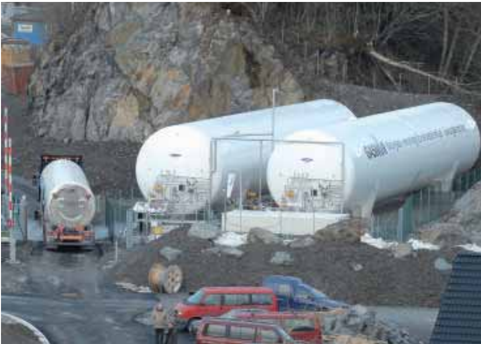
» Above: one of the two LNG tanks on board. Below: a fuelling station for the LNG ferry.
